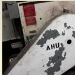
CHS Replace air handling units, C9, B3, A9
